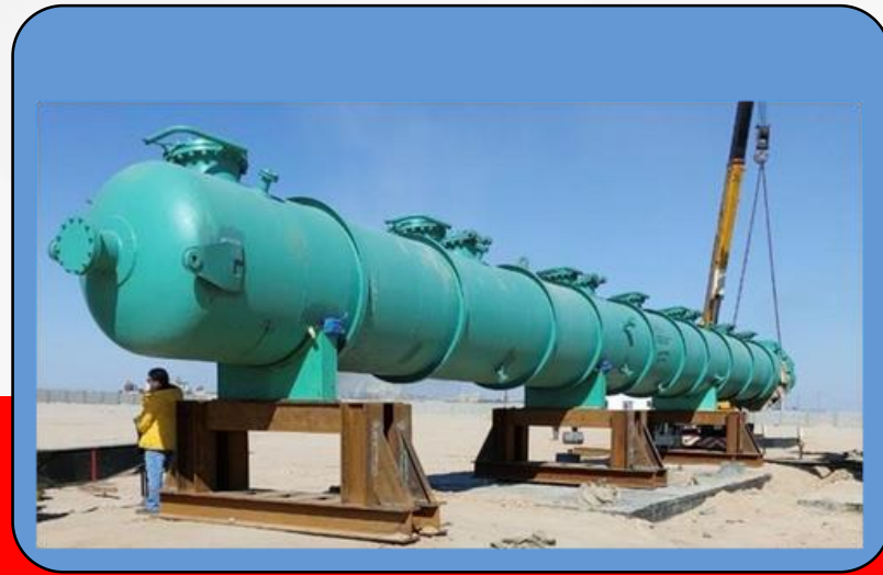
Crude Distillation Column
